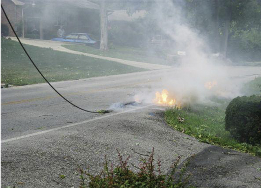
Figure 8.8 Downed power lines that are still energized can spark and cause fires. It is easy to tell that this line is still energized.
