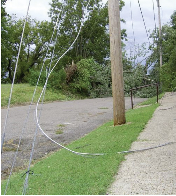
Figure 8.10 Sometimes fallen power lines appear to be harmless and de-energized because no arcs are occurring, when in fact they are energizing the ground and any other metal objects around them.
